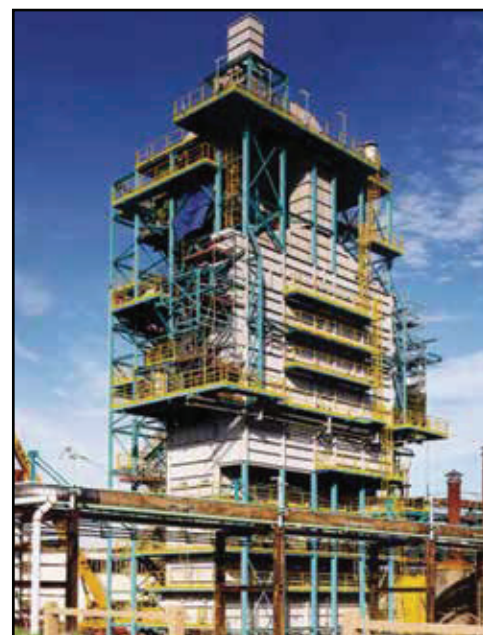
Ethylene Cracker Unit
